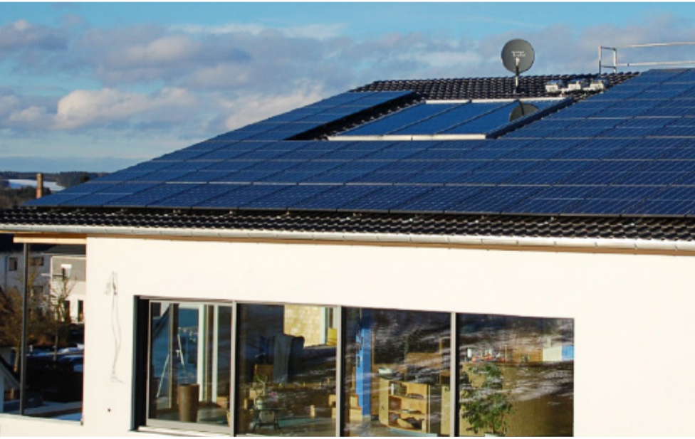
In March of 2019, this house powered by Q CELLS' solar panels in Augsburg, Germany, received the Federal Prize for Outstanding Innovative Achievements from the German Federal Ministry of Economics and Technology for achieving carbon neutrality through eco-friendly construction.
